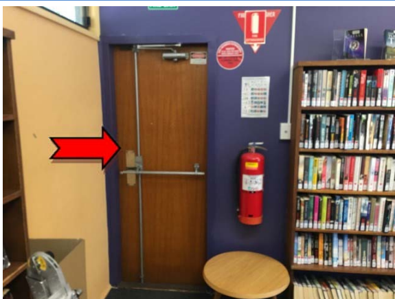
Photo 5. Interior, throughout, fire doors – suspected asbestos-containing fire door core.
