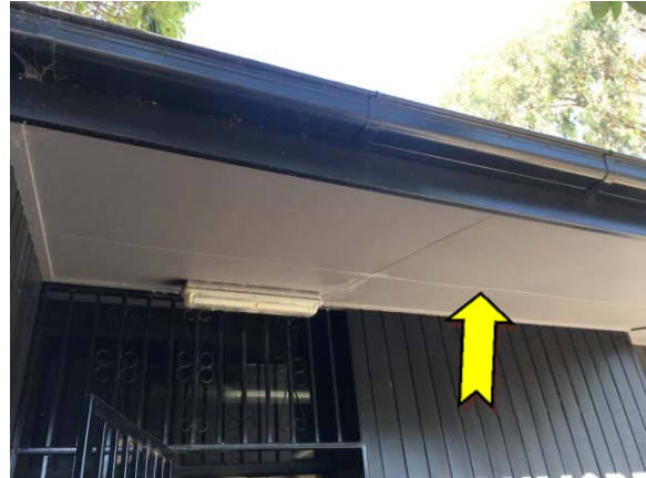
Photo 8. Exterior, throughout, awning – suspected lead-containing white upper paint systems.
