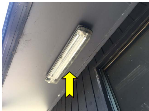
Photo 6. Exterior, throughout, single tube fluorescent light fitting – suspected PCB-containing capacitor.
