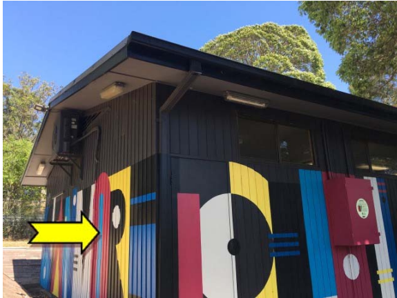
Photo 7. Exterior, throughout, walls – suspected lead-containing various coloured upper paint systems.
