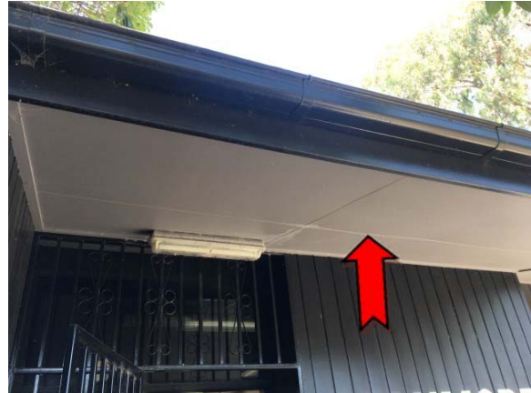
Photo 2. Exterior, main entrance, awning – suspected asbestos-containing fibre cement sheeting.
