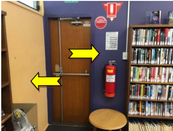
Photo 9. Interior, throughout, walls – suspected lead-containing orange and purple upper paint systems.
